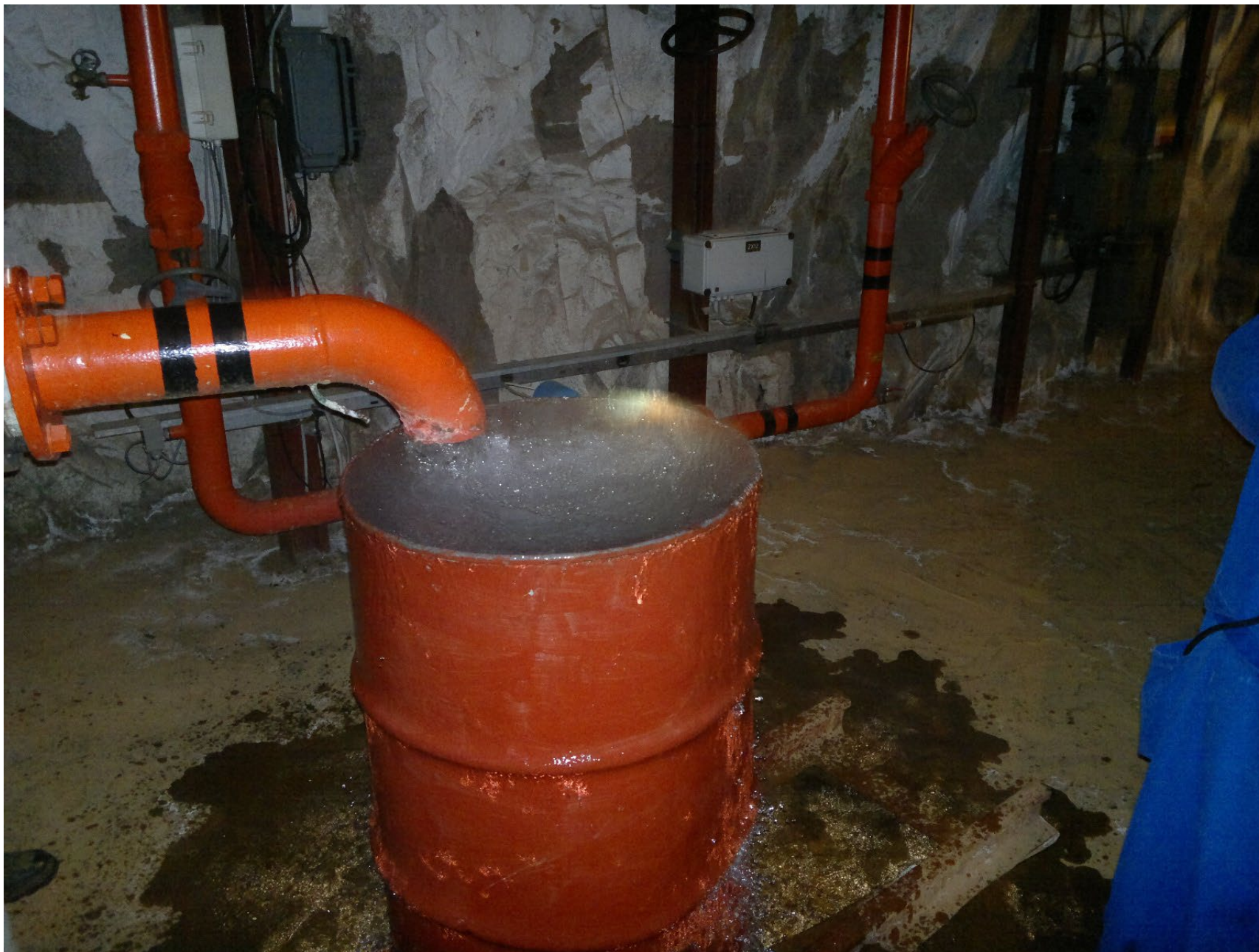
Fig. 5S. An open waste (drain) valve (photographed by the author T.Ř.).
